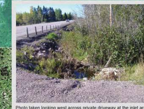
Photo taken looking west across private driveway at the inlet area of Tributary H immediately upstream of the existing road crossing, as well as the connection to the drainage ditch and entrance culvert for this laneway.
